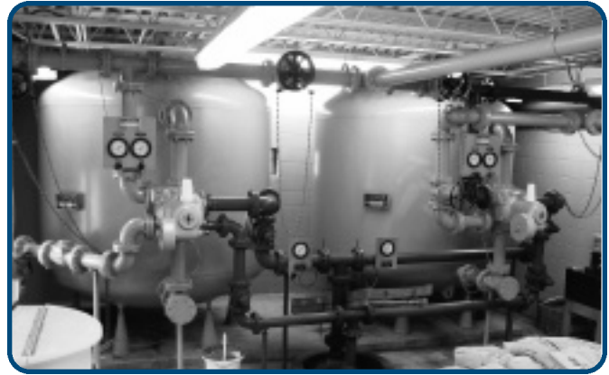
The Norton, Harding, Jimtown (West Virginia) PSD serves approximately 1,000 customers in two communities. On the right is a greensand filter and a carbon filter, used for low levels of phenols in the raw water, is on the left. This plant has two additional greensand filters that remove 3.3 mg/L iron and 0.4 mg/L manganese at a pH of 6.5.
