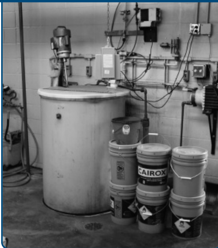
This photo shows a typical setup to feed potassium permanganate consisting of a tank, mixer and feed pump.
