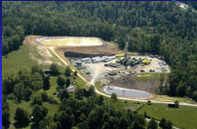
Pads can be 5+ acres – but one pad may support drilling multiple horizontal wells.
